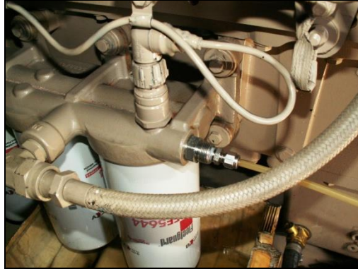
Fuel filter with sample port for contamination monitoring
